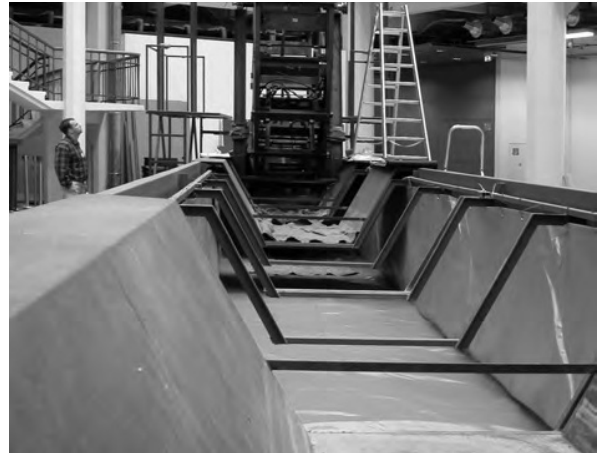
Fig. 5. Modifications in 1997. Installation of a foil tank (in blue) in the substructure to ensure against leaks. Courtesy of ZKM.
